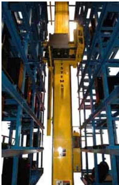
NorthStar System stores batteries up to 10 high
