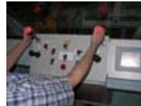
Lighted wand safety switches
